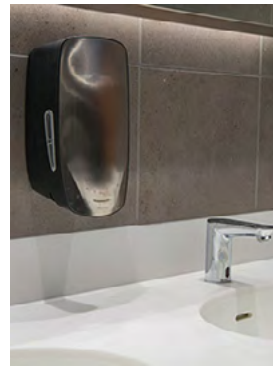
Soap Dispenser in a restroom.
